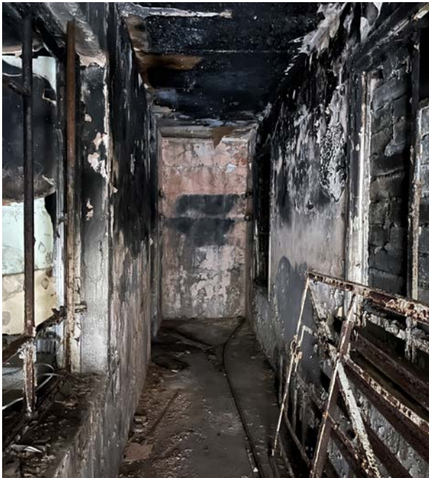
Figure 37 - Fire damage in Barnhall House
