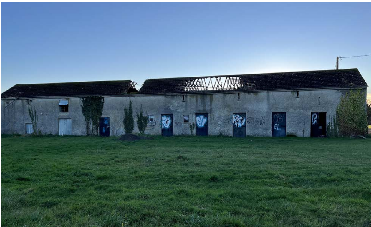
Figure 46 - The east-west stable building in advanced state of dereliction
