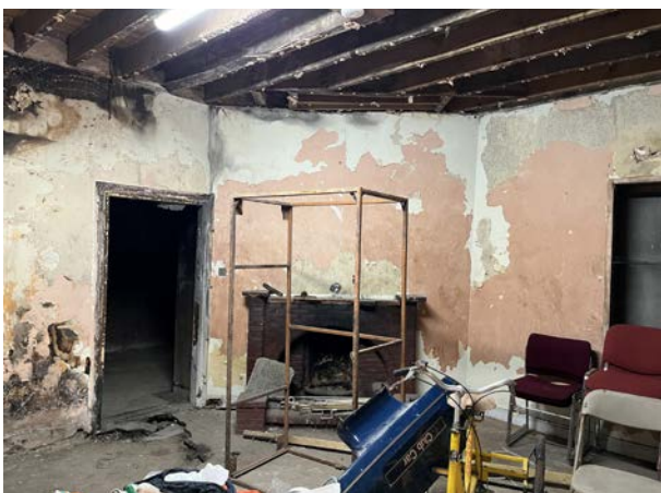
Figure 38 - Derelict interior of the house
